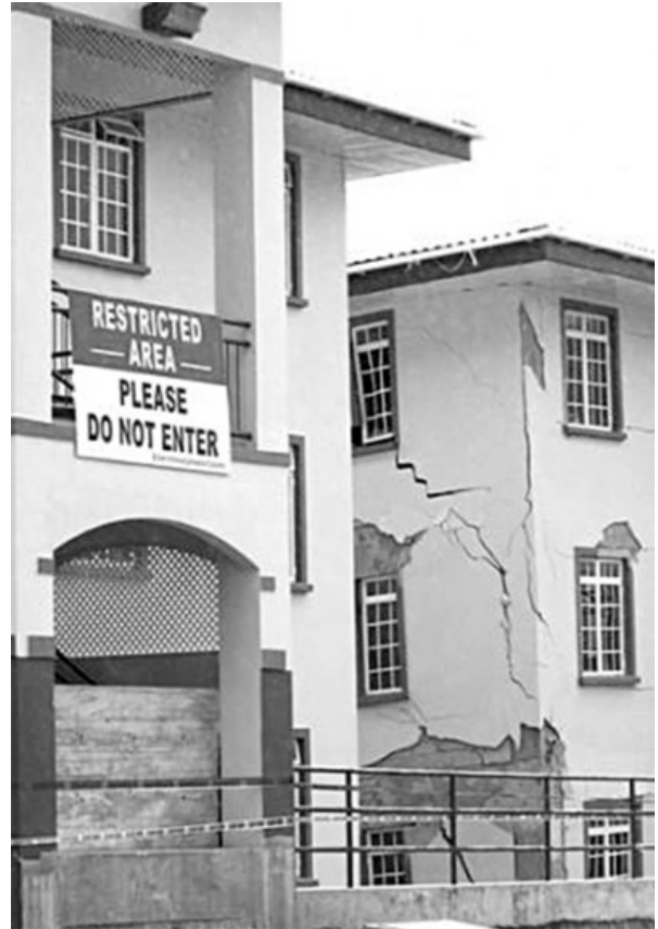
Las Alturas buildings cracked. Courtesy T&T Guardian.
